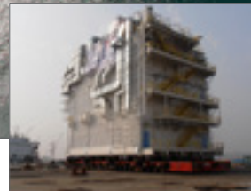
FPSO for Libra Field e-House electrical distribution module being installed on FPSO topside
